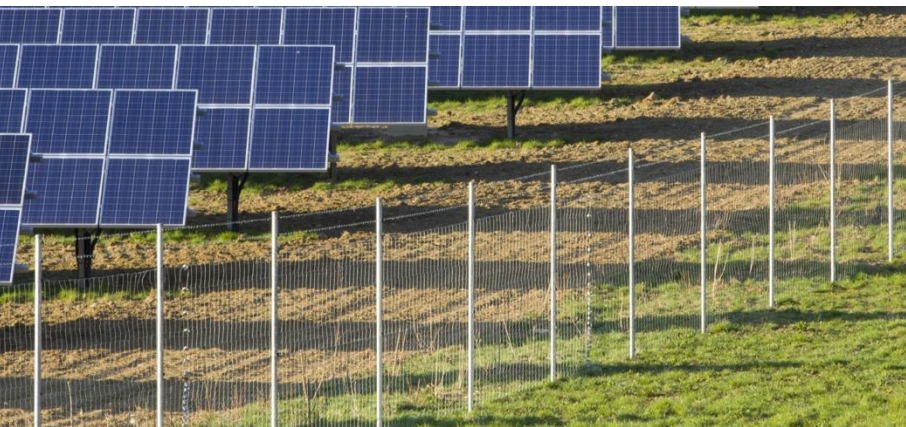
Example of a deer fence around a solar site
