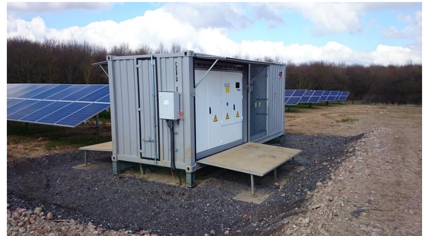
Example of a containerised inverter
